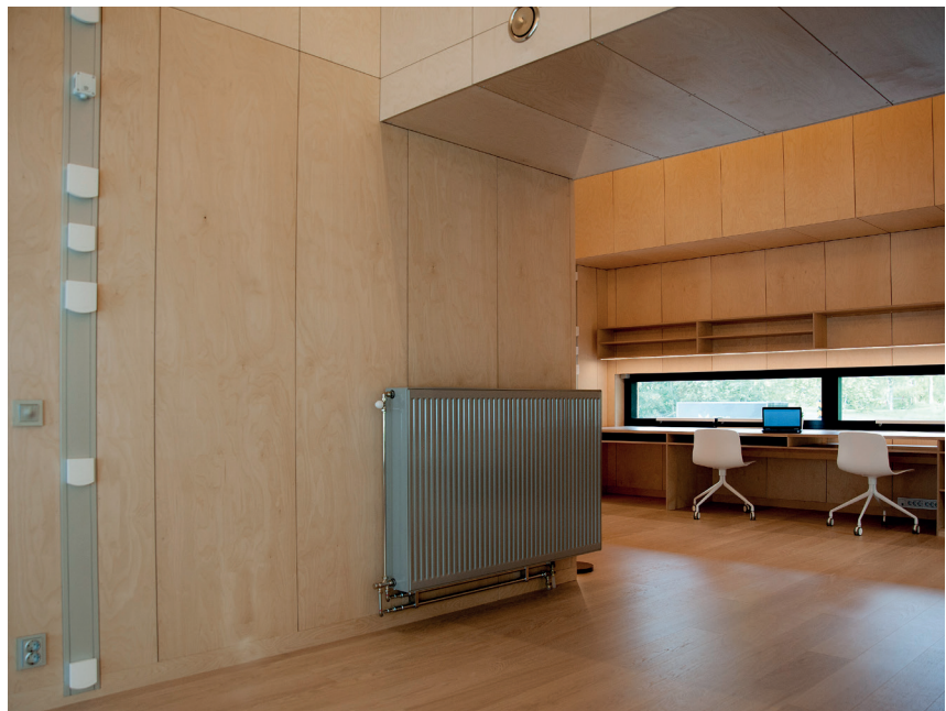
Figure. The ZEB Living Lab's radiator is placed on an inner wall in the Living room. Rated heating power is ca. 2800 Watt at 55/50 °C su.
