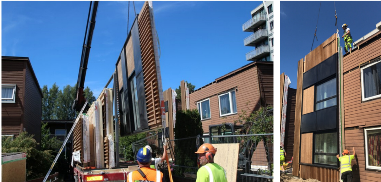
Figure 12: Mounting of elements with integrated PV and ventilation ductwork, Oslo Demo Haugerudsenteret
